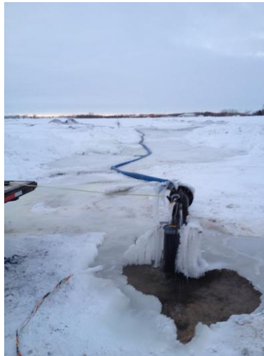
Figure 26 – The South Production well and discharge hose heading southwards off the site.
