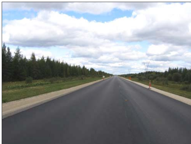
Highway 6, east of the proposed project area, looking N: Large cleared shoulders on either side of road have created suitable habitat for some invasive plant species (refer to observation site MN 22).
