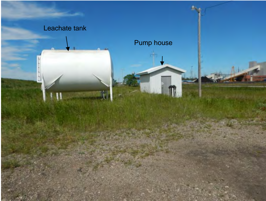
Photograph 9: Former leachate tanks and pump house with flow meter located along north property boundary (11-Jul-14).
