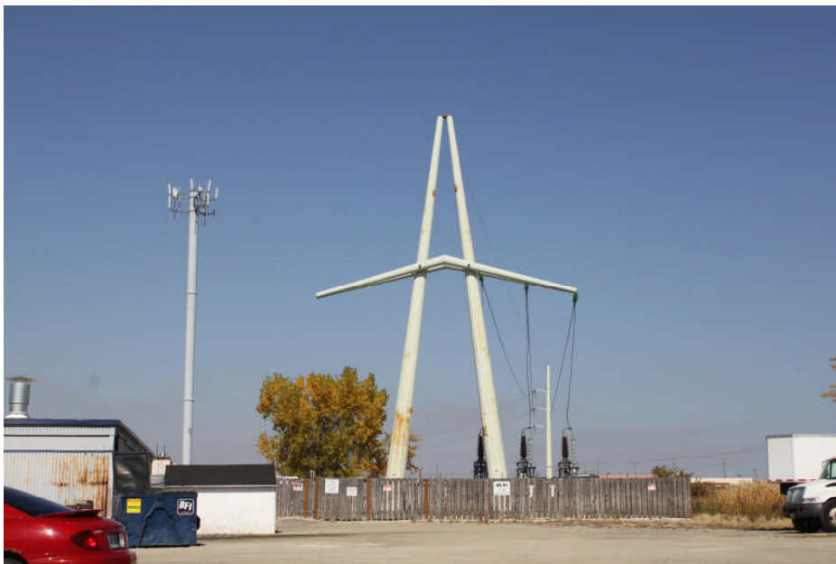
Photo 6: St. James to St. Matthews Terminating Structure
