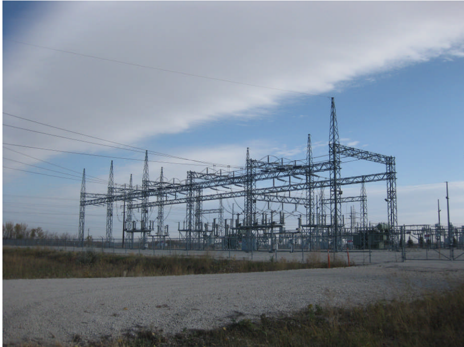
Photo 3: Example of 115 kV Air Insulated Switchgear
