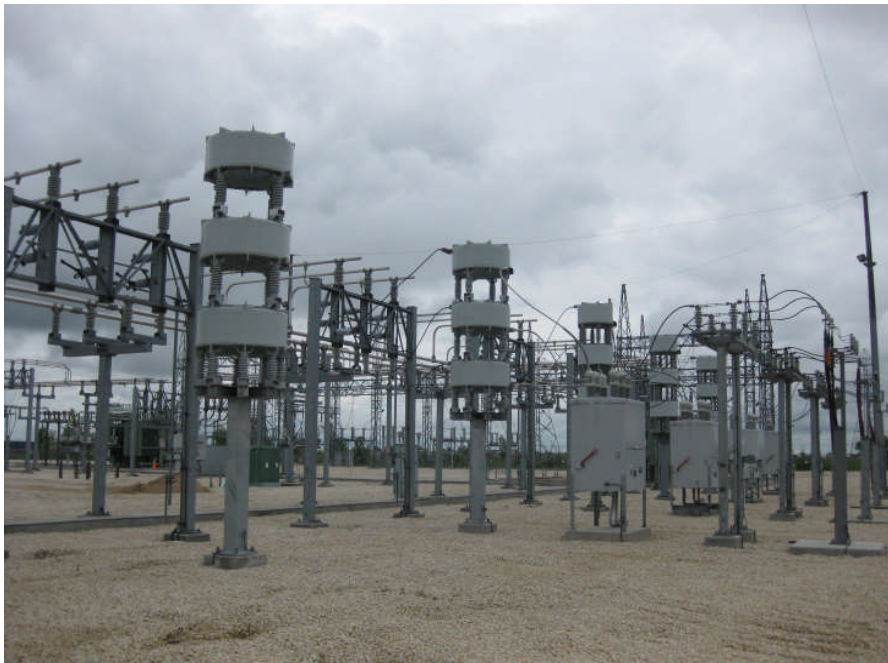
Photo 4: Example of 24 kV Outdoor Equipment and Structures
