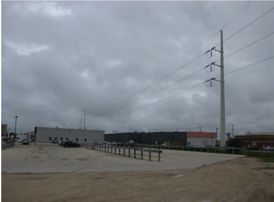
Photo 5: Existing RS51 115 kV Transmission Line
