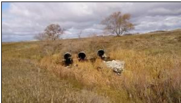
Photo 4-3: Outlets from control structure on Bosshill Creek north of PR 257.
