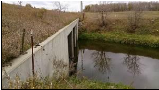
Photo 4-21: Gopher Creek at north PTH 1 service road crossing, looking west (700 m from outlet).
