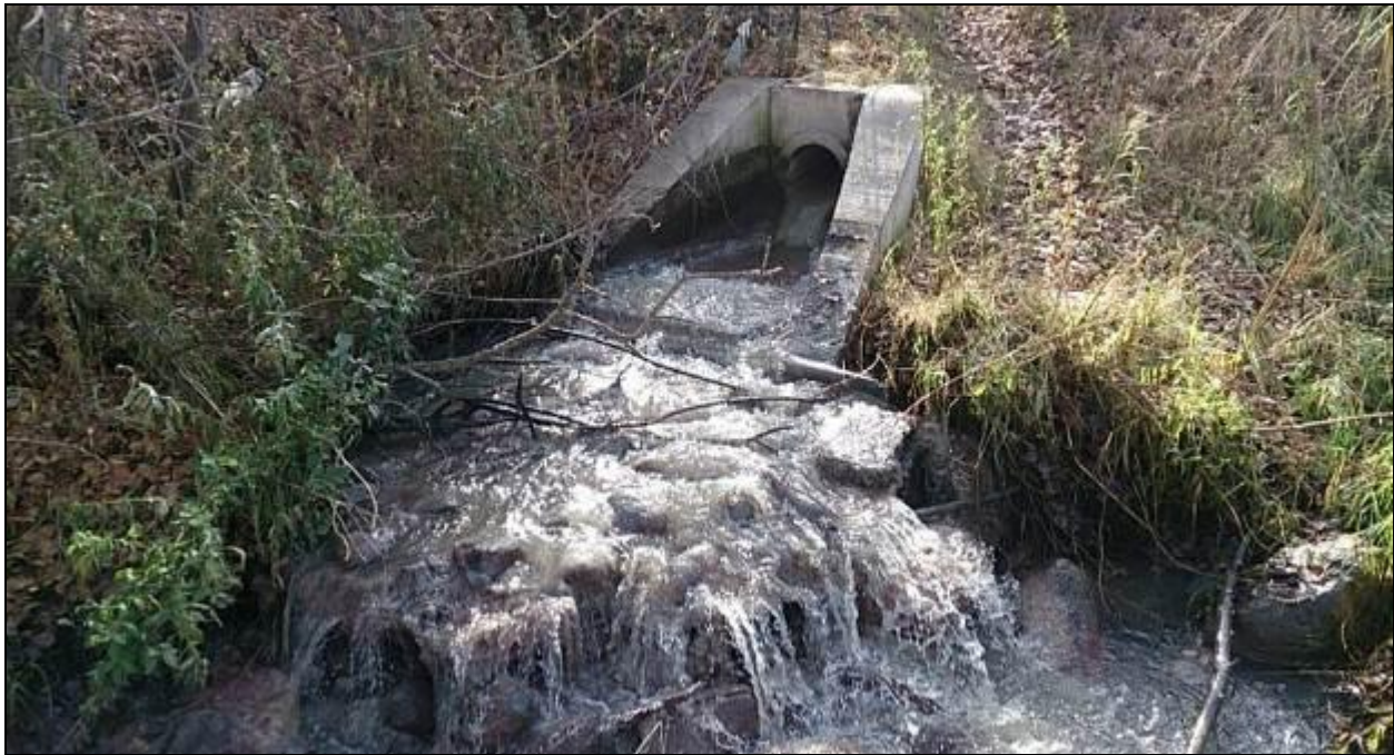
Photo 2-4: End-of-pipe discharge of treated effluent from existing Virден WWTP into the surface drainage channel.
