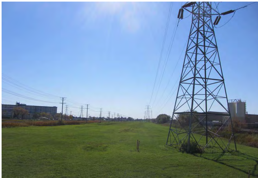
Photo 04. Southwest view showing cut grass along ROW and existing transmission lines.
