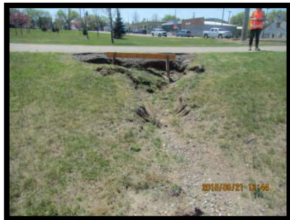
Photo 10 – Looking at an erosion trough on the north side of the pedestrian path (south of grassed secondary slope), May 21, 2015.
