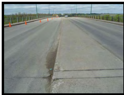
Photo 1 – Looking north at Site#2582-00 on PTH 1A, May 29, 2013 (Inspection Report).
