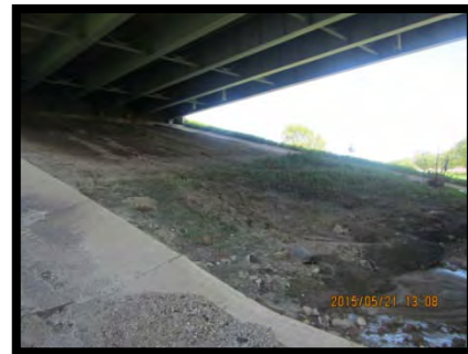
Photo 12 – Looking northeast under the structure at erosion from the northwest bank, May 21, 2015.
