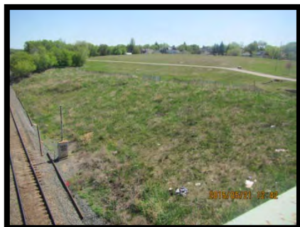
Photo 7 – Looking (southeast) at the secondary grassed bank south of CP rail, May 21, 2015.
