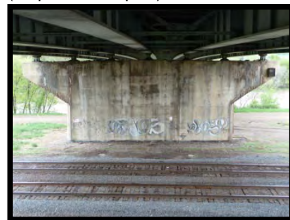
Photo 6 – Looking (north) at the southern pier near CP rail, May 29, 2013 (Inspection Report).
