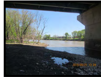
Photo 5 – Looking (east) under the structure at the northeast bank from the pedestrian path, May 21, 2015.
