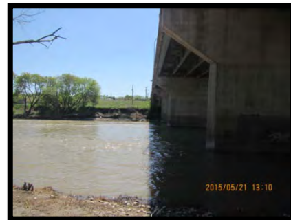
Photo 6 – Looking (south) at the east side of the structure and the Assiniboine River, May 21, 2015.
