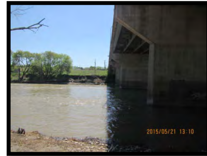
Photo 6 – Looking (south) at the east side of the structure and the Assiniboine River, May 21, 2015.
