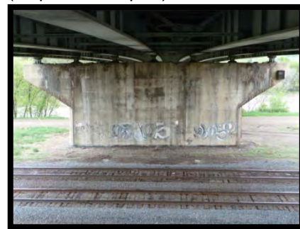
Photo 6 – Looking (north) at the southern pier near CP rail, May 29, 2013 (Inspection Report).
