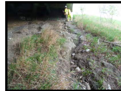
Photo 9 – South embankment with severe erosion trough, May 29, 2013 (Inspection Report).
