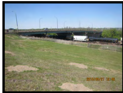
Photo 11 – Looking (northwest) at the downstream elevation (approx. 50 m downstream) and CP rail, May 21, 2015.
