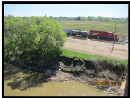
Photo 4 – Looking (southeast) at the southeast bank, CP rail and severe bank erosion from structure, May 21, 2015.
