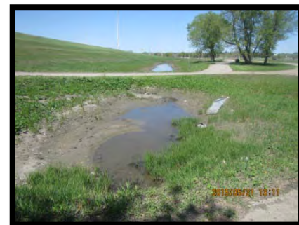
Photo 12 – Looking (north) at the drain/water that intersects the Assiniboine River downstream Site#2582-00, May 21, 2015.
