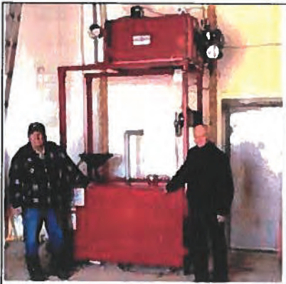
Ron Benson, Executive Director of MARRC with Solomon Mason, Project Manager with St. Theresa Point standing in front of the used oil burner installed at the Fire Station
