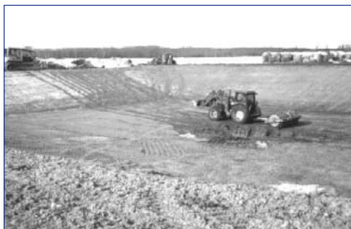
Final stage of the construction of an earthen storage: compacted with a sheepsfoot packer
