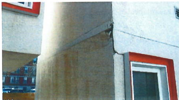
Fig. 3: Damaged wall and stucco due to jacking.
