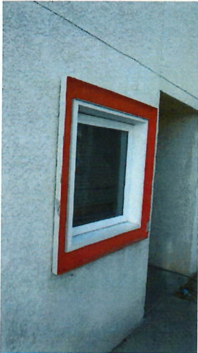
Fig. 14: Another example of peeling trim.
