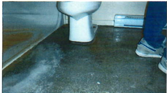
Fig. 5: Toilet raised off floor due to drain lifting.
