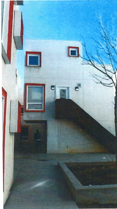
Fig. 17: Exterior example of cantilever dropping at outer edge.
