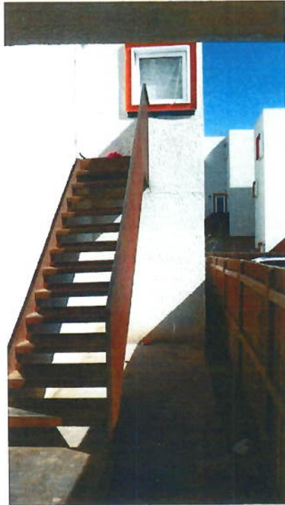
Fig. 11: Example of corroding stairs.
