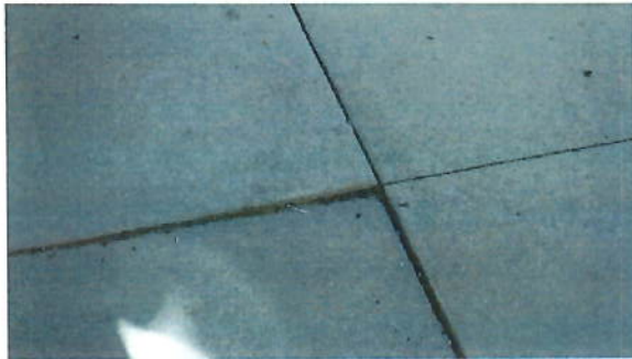
Fig. 7: Example of uneven sidewalk.
