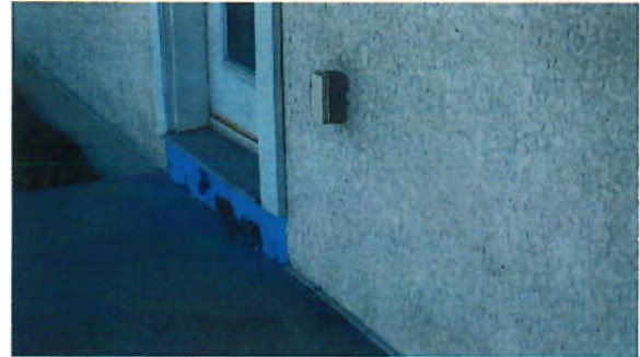
Fig. 9: Example of missing stucco below door.
