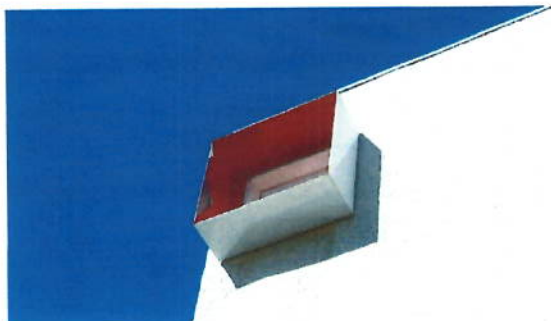
Fig. 13: Peeling window trims.
