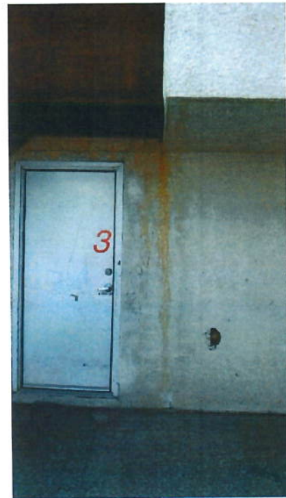
Fig. 12: Example of staining occurring on stucco due to stair corrosion.
