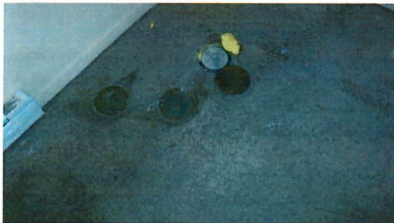
Fig. 6: Floor drain raised out of floor.
