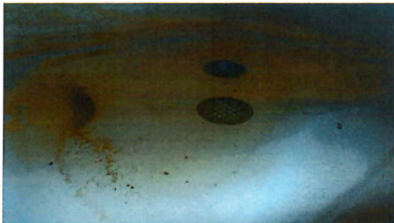
Fig. 4: Shower drain lifted out of shower floor.
