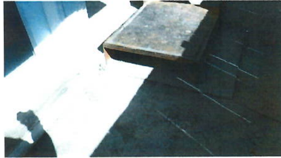
Fig. 8: Multiple elevations to walk through: concrete pad to left of metal platform, metal platform, lower concrete slab, uneven/unmatched sidewalk.
